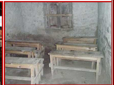
Decay of the school in Lipni
